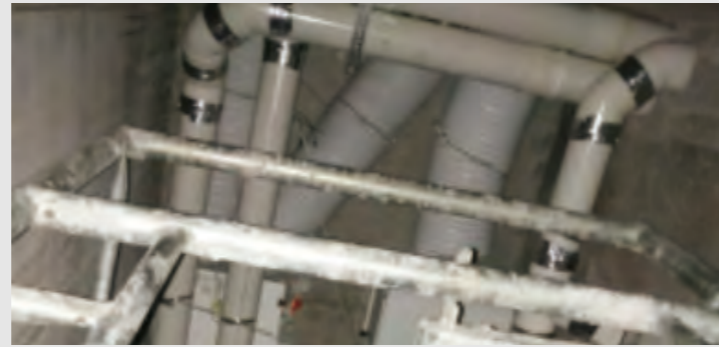
02-The quality of the pipeline material is poor. ❌
