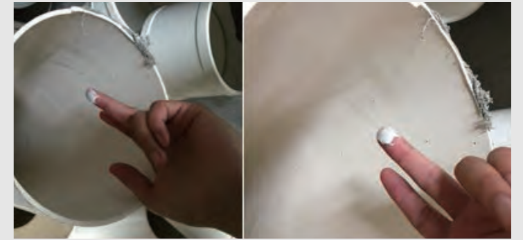
04-Accumulation of dust inside the pipeline ❌
